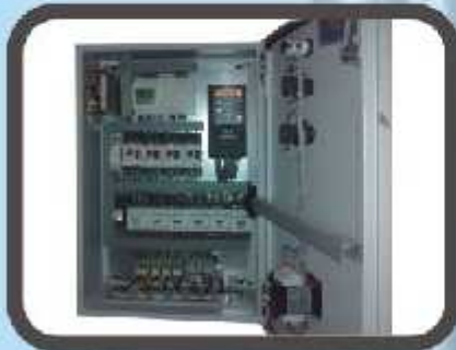
Control Panel (PLC/VFD)
